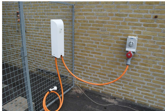
(d) Temporary EVSE installation for testing. It draws 63A from a CEE outlet.
