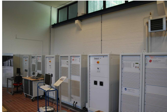
(d) Three-phase 150kW power amplifier connected to the motor. The cable to the motor is quite long and must be taken into account.
