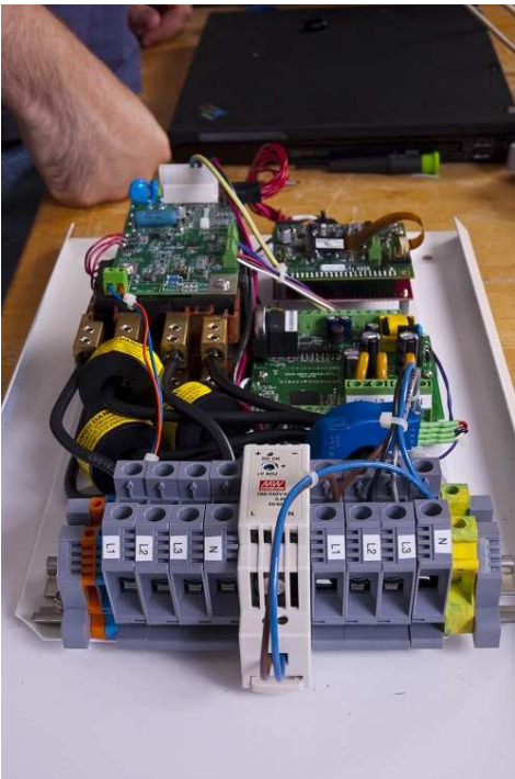
(c) Finished three-phase EVSE.
